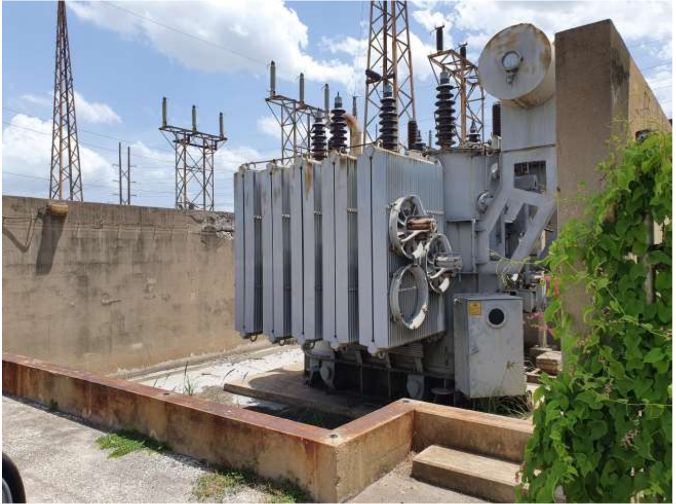
1 st PCB Transformer at Hunts Bay – oil already drained (N.B. Area is de-energized)
