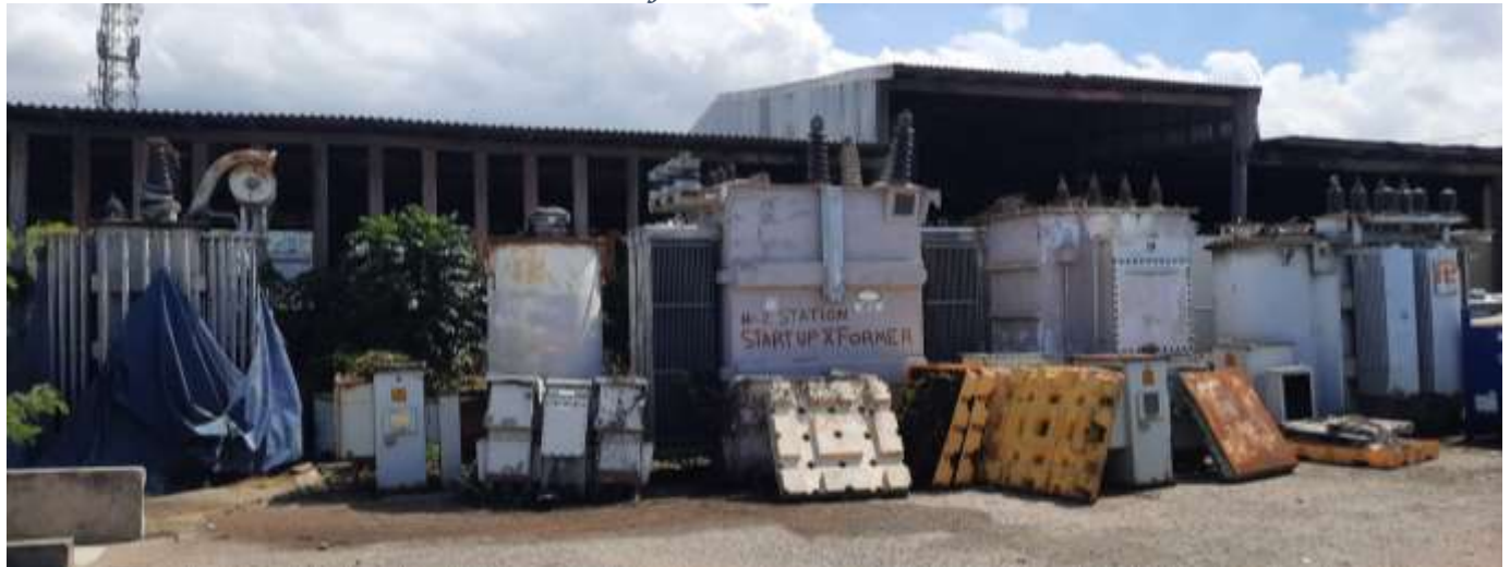
Some PCB transformers and Switches
